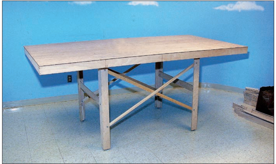
A simple table can be built from dimensional lumber or, in this case, plywood ripped to 3"-wide strips. A plywood or foam tabletop is a good starting point.
