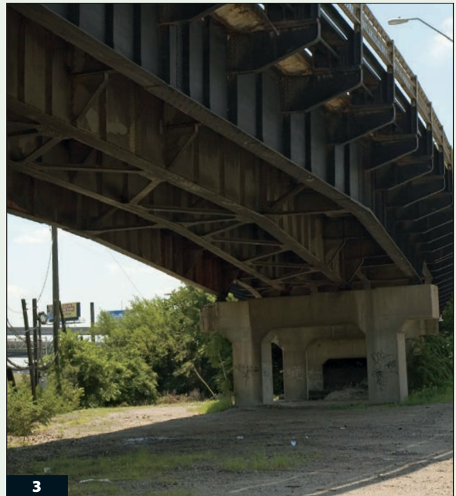
Upon closer inspection, you can see that the girders are straight while the deck is curved.
