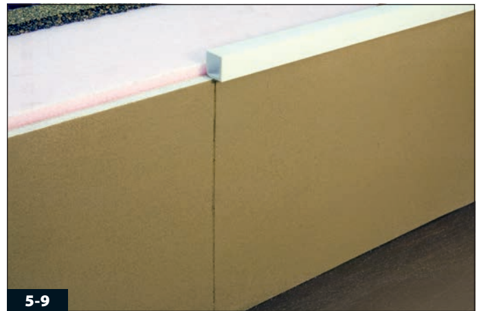
5-9 The cap should be painted before applying it to the top of the walls. (It is shown here unpainted for clarity.)
