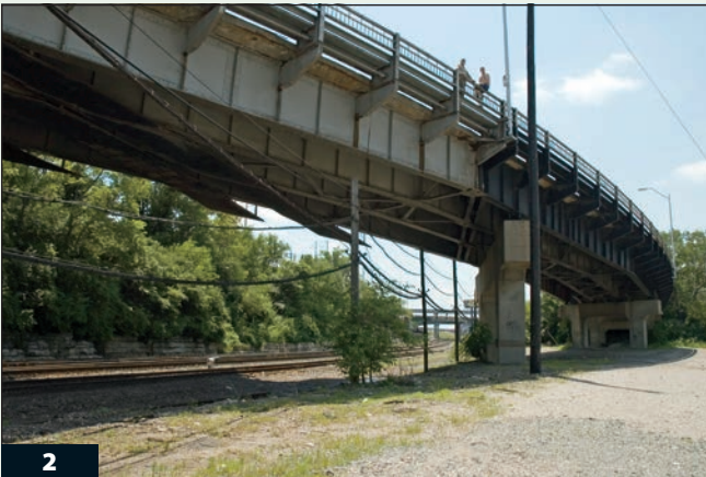
Looking from the opposite direction, you still might assume that the girders are curved.
