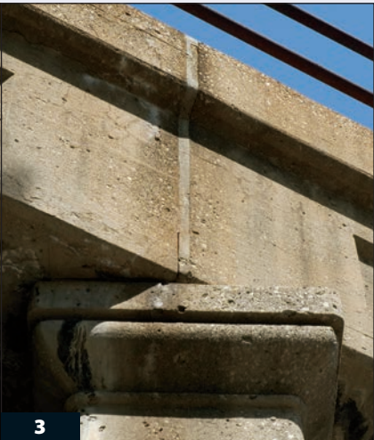
The rough concrete texture results more from a mottled appearance than an actual bumpy surface.
