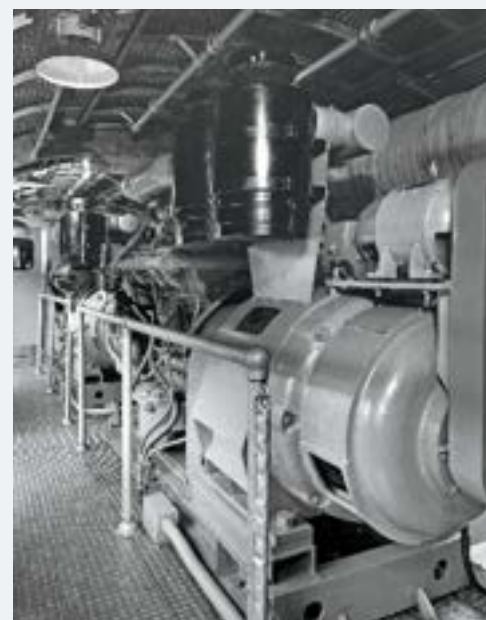
Adjacent to the kitchen, two diesel generator sets supply electricity to the train. PBB
