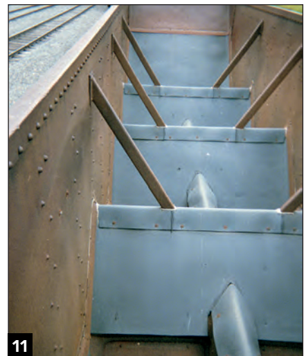
11 This interior view of BGSX 122558 shows the repairs that were made to the quad hopper. William Phalen, Cody Grivno collection
