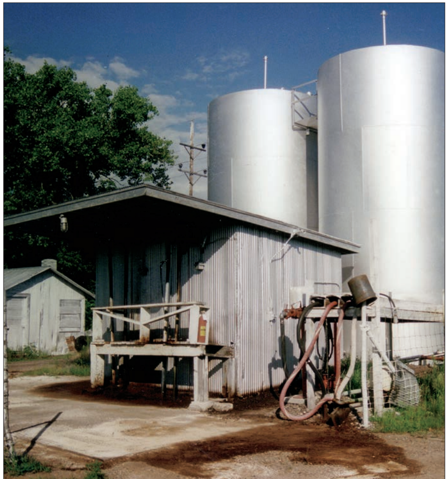
Rail-served bulk oil dealers can be found across the country, and the tanks, structures, and fittings offer a great deal of modeling and detail potential.
