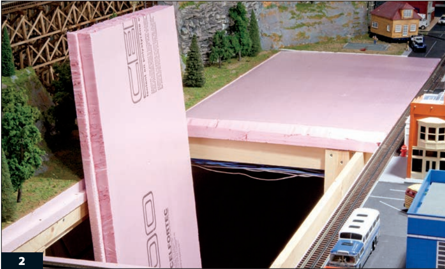
2 Lightweight foam insulation board is the key to building a concealed access hatch that's easy to remove yet rigid enough to support scenery and structures.
