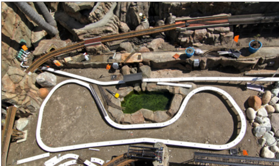
4. The railroad under construction. Track is in place on some of the lines, while others are still being built. White PVC is used as a road base.
