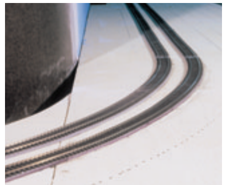
Fig. 6 TOPPER TAPE ON CURVES. The protective skin has to be removed to bend the tape around curves. It's important not to stretch the tape on curves so it will maintain an even thickness. Once the tape is in place, Chuck lays a bead of adhesive caulk on the tape before installing the track.
