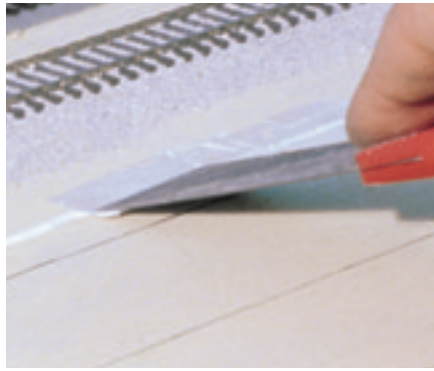
Fig. 2 SPREADING CAULK. Chuck lays about an \frac{1}{8} " bead of DAP All Purpose Adhesive Caulk and spreads along the pencil guideline. A thin layer of caulk is sufficient for holding the track in place. If the material squeezes up between the ties, you're using too much.
