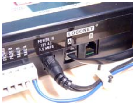
Fig. 10 Loconet. A cable connects the plug panel to the Loconet socket on the back of the command station.
