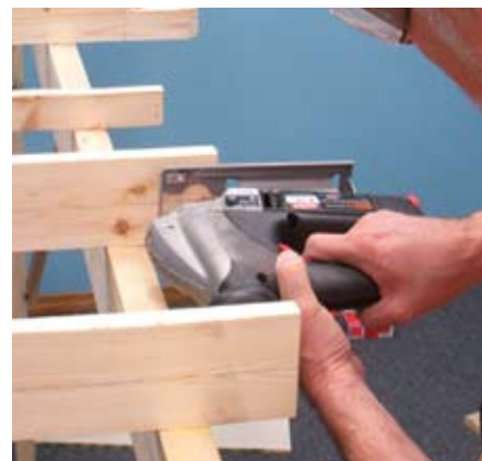
Fig. 9 Lowering the joists. After marking the edge of the creek bed and wash on the joists, Stener measured down 2" and then used a saber saw to cut the joists. These slimmer, cut-down joists support the base for the plywood creek.
