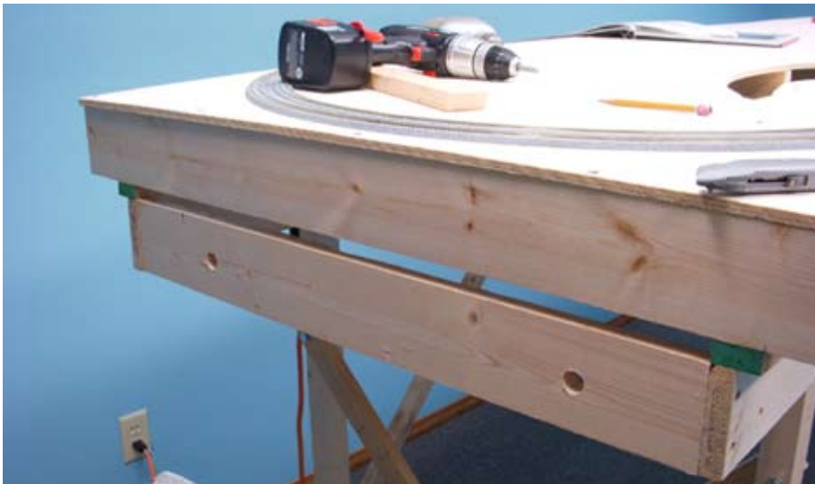
Fig. 4 Reinforcing the ends. Dick and Stener realized that the layout would be lifted at the ends, and that the fascia would extend to the bottom of the girders. They added 1 x 4s at each end of the layout to serve as gripping points.
