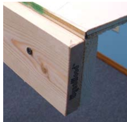
Fig. 7 Double the joist. Where the additional 12" of plywood was added to the end of the layout, another joist was needed for support. It's the same length as its mate, and Dick and Stener secured it with glue and screws to the L girder.
