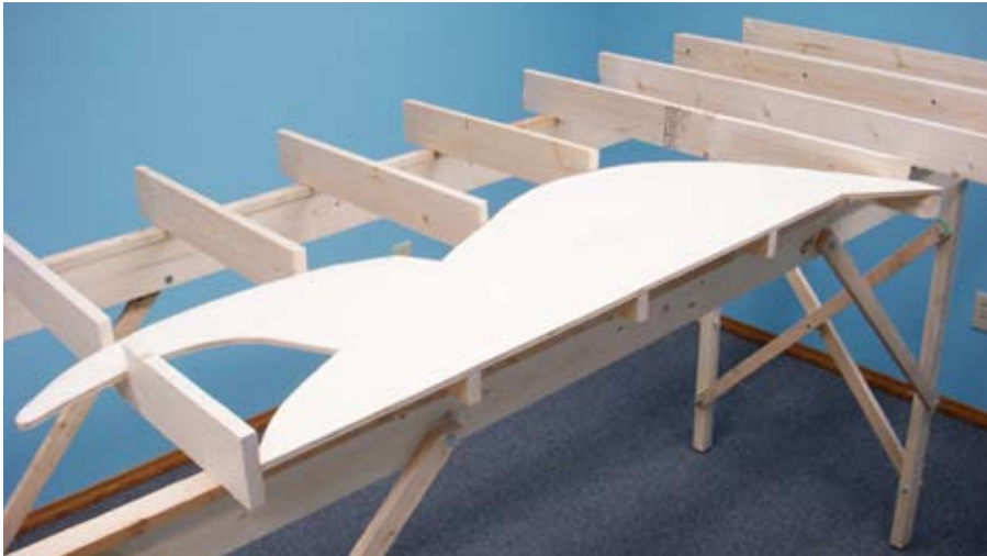
Fig. 10 Below-grade scenery. Here the grade-level plywood has been removed and the wash bed plywood put in place. A few additional supports were needed to keep the plywood from sagging between joists.
