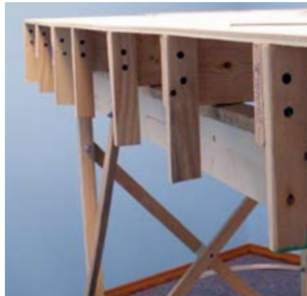
Fig. 12 Fascia fine points. Dick and Stener used glue and screws to attach vertical 7" lengths of 1 x 2 to the side of the joists to support the layout's hardboard fascia.
