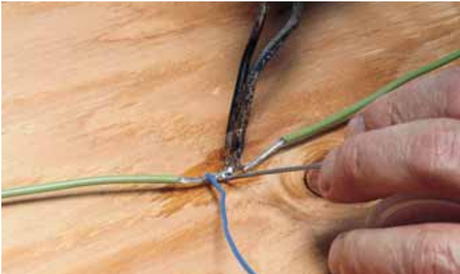
This simple Tee splice connects wires under a layout.
